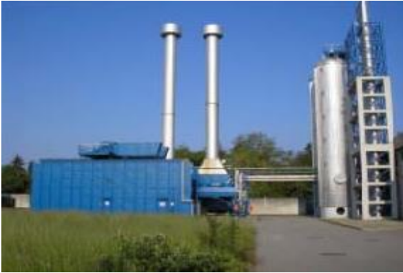
TURBINA A GAS GAS TURBINE TURBINE A GAZ
