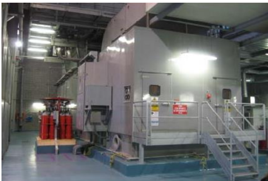
TURBINA A GAS
